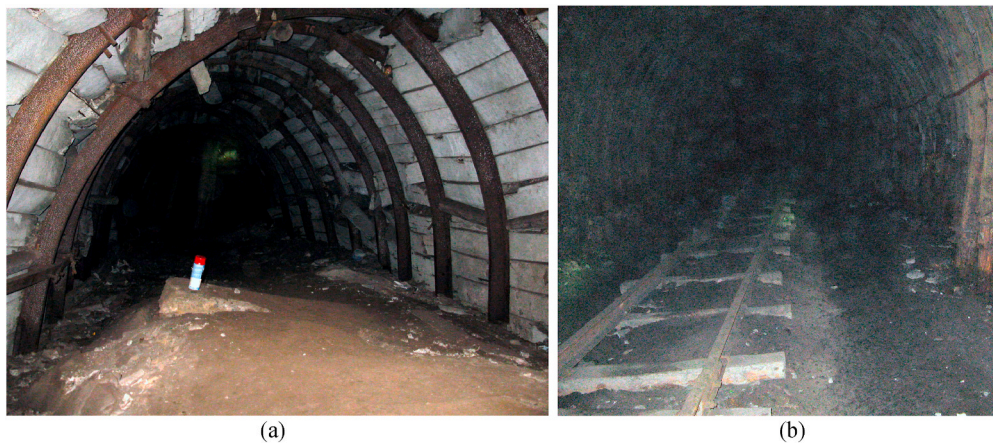
Fig. 21. Floor heave. (a) in ventilation cross-cut after using a concrete beam; (b) in main ventilation cross-cut after grouting with depth of reinforcement 1.75 m.
